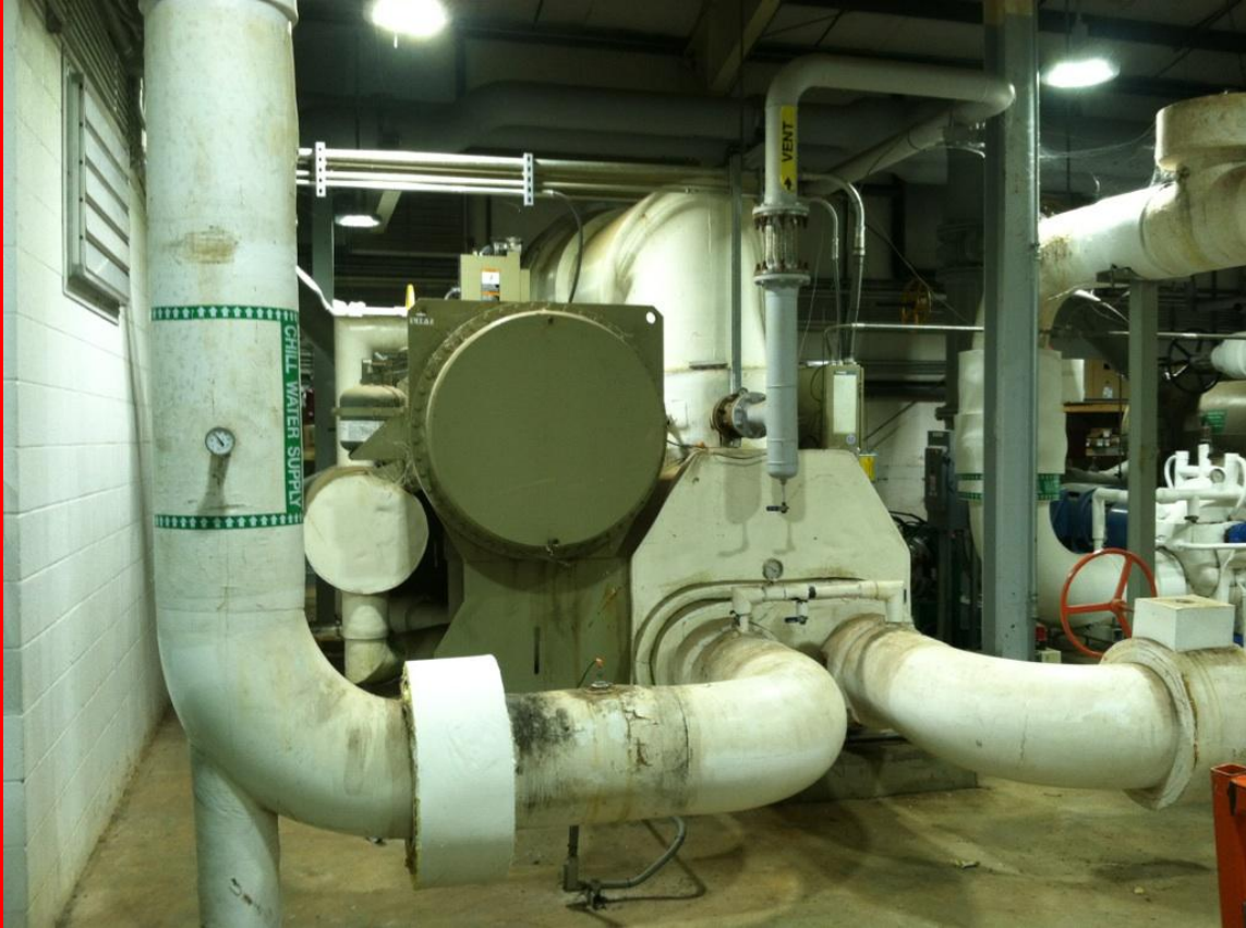
Existing Chiller To Be Replaced
