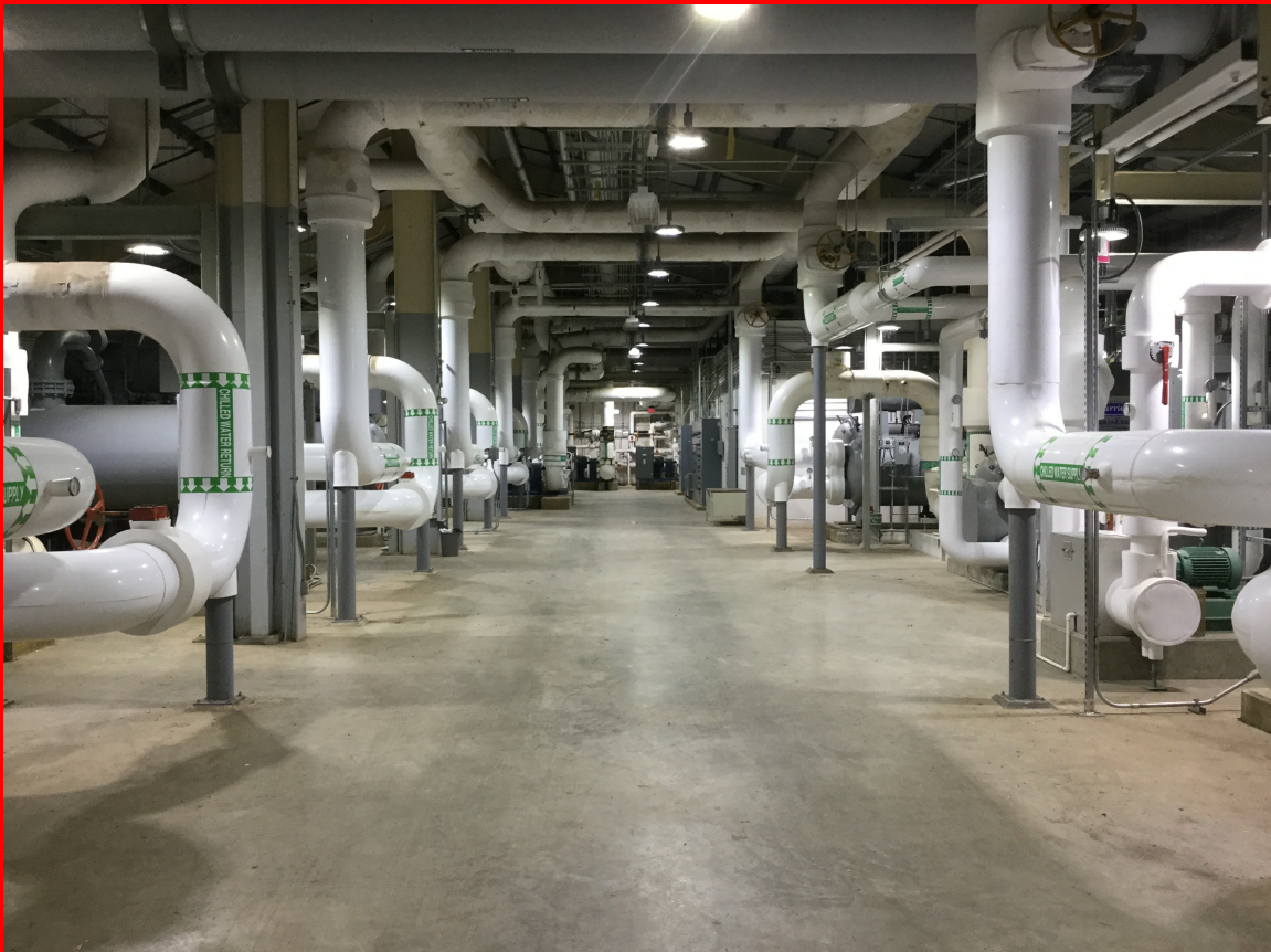
Chiller Plant After All Chillers Changed Out
